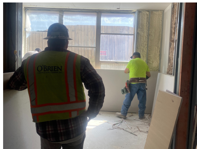
Drywall is going up inside of the St. Matthews school. Image courtesy of Rachel Pisano
