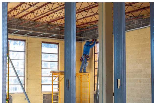
Framing inside the St. Matthews gymnasium is nearing completion. Image courtesy of Jim West
