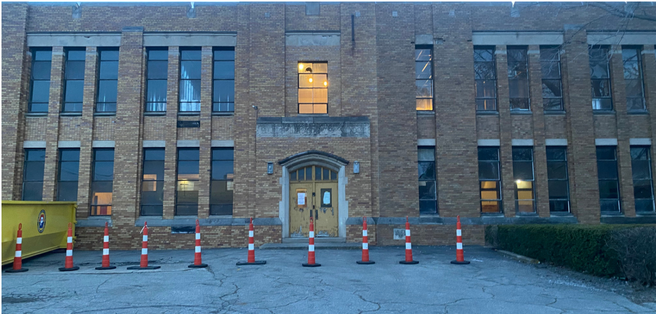
Renovation of the former St. Mathews school is fully underway. Image courtesy of Jeffrey D. Lewis II
