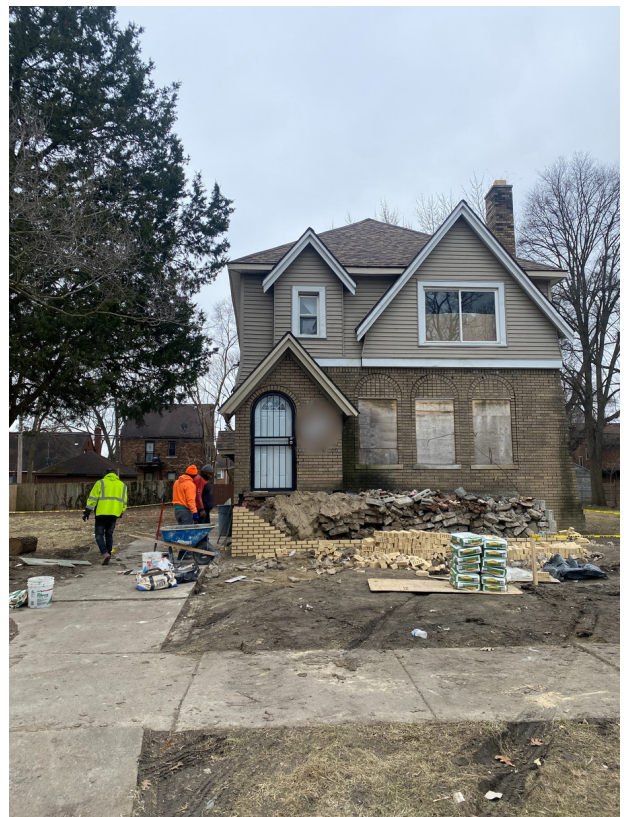
Exterior renovation work happening at the first home on Three Mile. Image courtesy of Rachel Pisano
