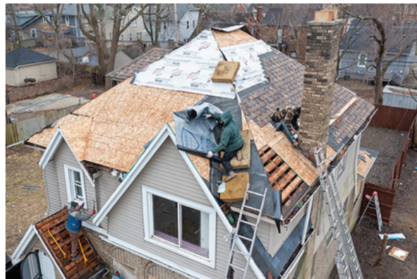
A complete install of a new roof. Image courtesy of Jim West
