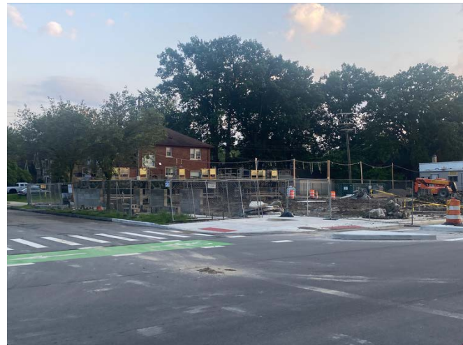
The exterior wall for The Ribbon development is starting to rise. Image courtesy of Jeffrey D. Lewis II
