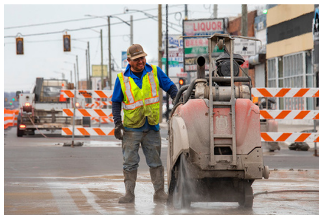
A crew member uses an industrial utility concrete saw on the south side of East Warren. Image courtesy of Jim West
