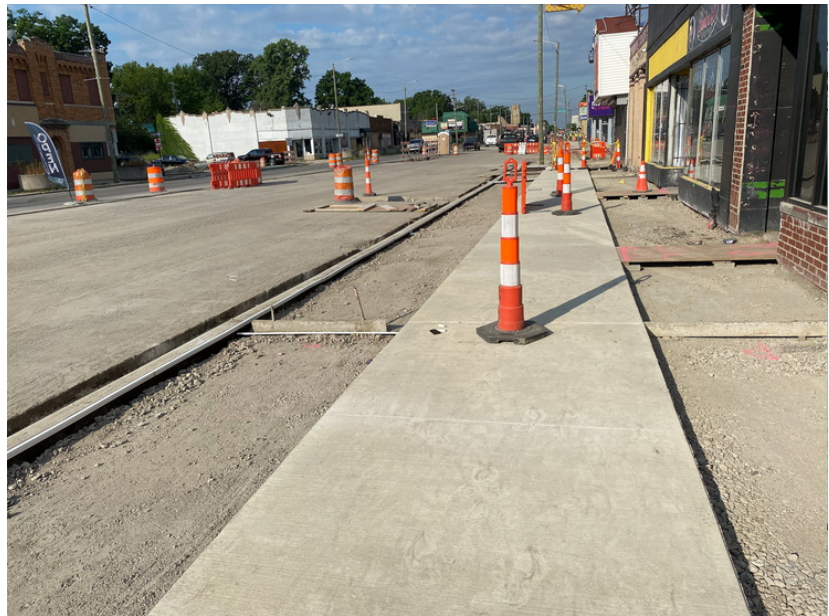
As a part of the streetscape project on East Warren, new sidewalks have been installed. Image courtesy of Jeffrey D. Lewis II
