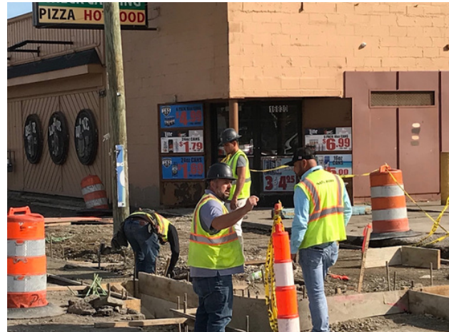
Construction shifts to the south side of East Warren. Image courtesy of Susan Newell
