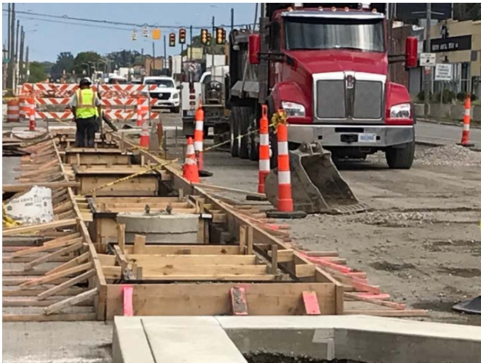
Framing is set for the new raised platforms set to separate the bike lanes from the parking lanes. Image courtesy of Susan Newell
