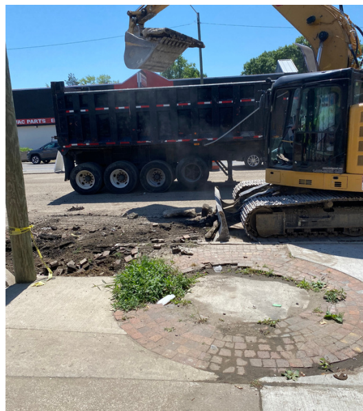
A sidewalk slab is placed in a dump truck. Image courtesy of Jeffrey D. Lewis II
