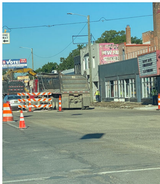
Construction is in full motion along the East Warren corridor. Image courtesy of Jeffrey D. Lewis II
