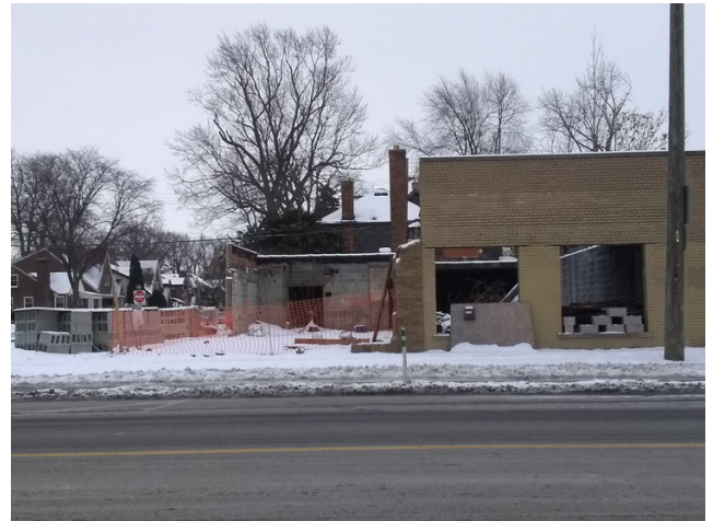
Collapsed building owned by Sarmed Ridha. Image courtesy of Eric Dueweke
