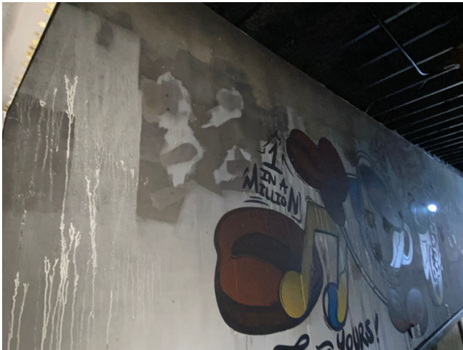
The fire severely damaged the customized mural. Image courtesy of Jeffrey D. Lewis II
