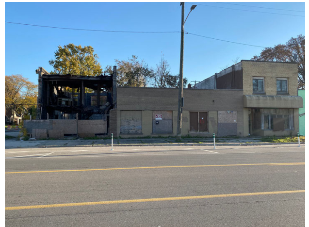
The partially demolished structure at 16134 E. Warren. Image courtesy of Jeffrey D. Lewis II
