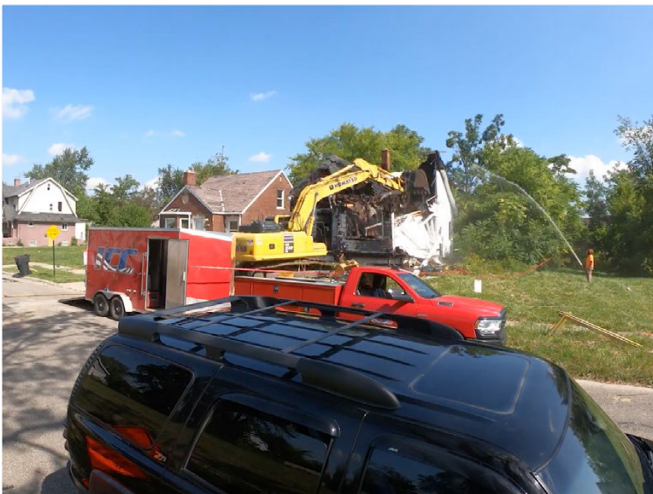
The long overdue demolition of 4350 Nottingham St. took place recently. Image courtesy of Nicolas Hall
