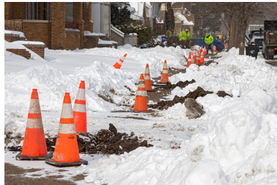
Sidewalks partially removed to replace the cast-iron gas mains. Image courtesy of Jim West
