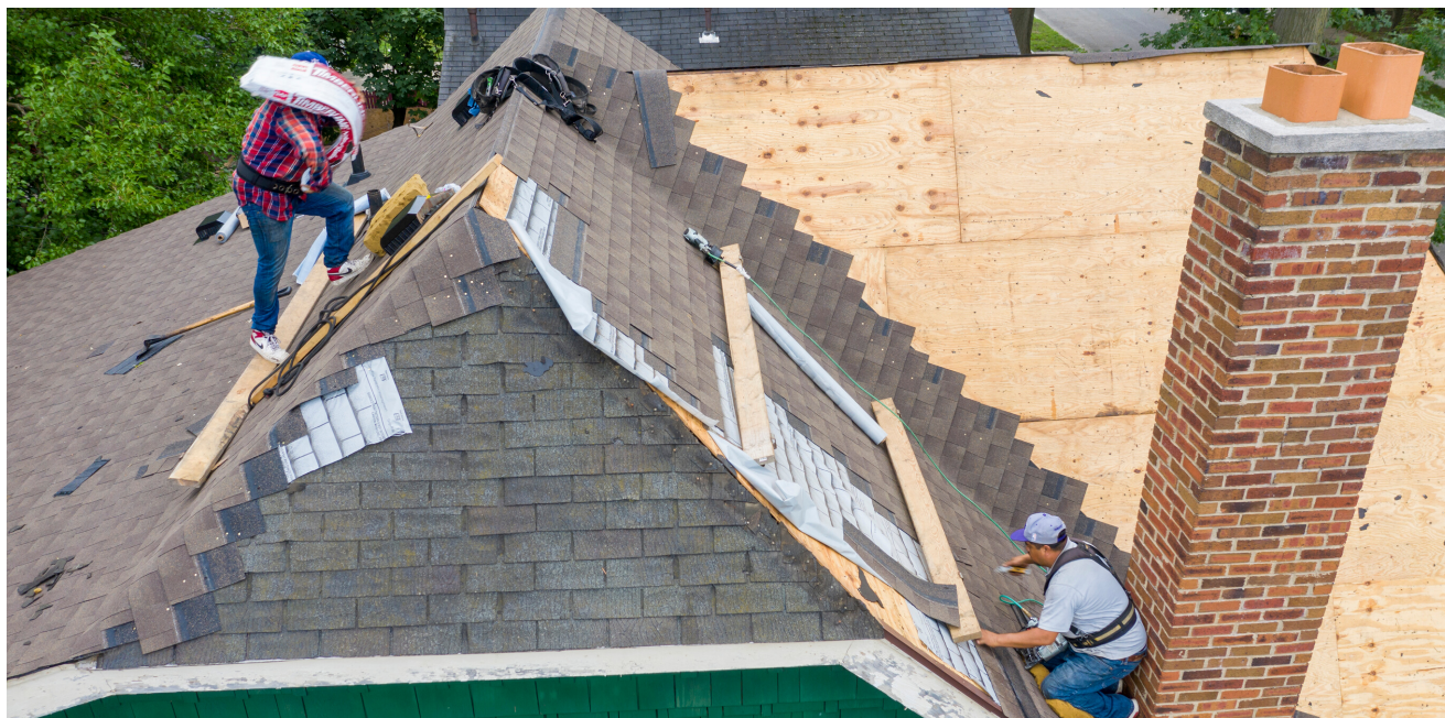
A new roof installation is just one of the many repairs the NIP Grant can provide. Photo by Jim West
