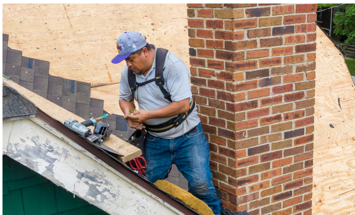
A roof installation is in full effect for this home. Photo by Jim West
