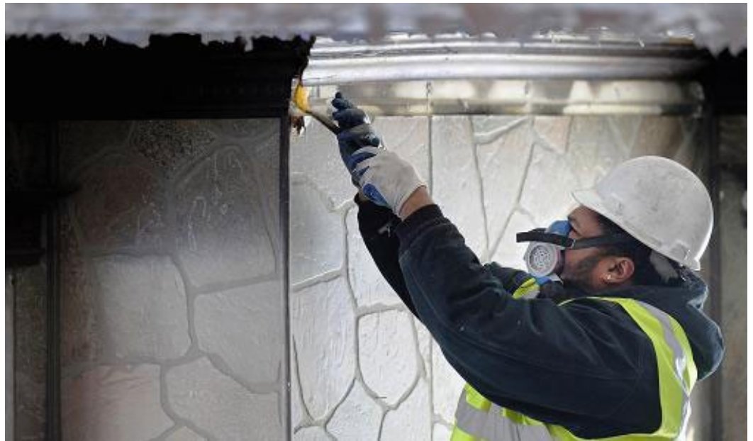
A construction worker pulls down old wood molding at an abandoned house on Elmhurst Street in Detroit, Michigan
